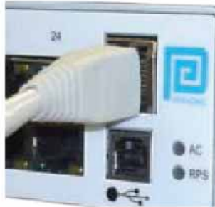
Figure 8: NIC Cable Connected*
